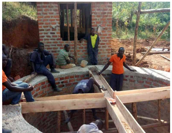
RIGHT: Work progresses on a water tank and pump house in Uganda.
